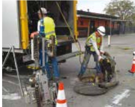
Deployment of the SewerVUE Surveyor at the Del Norte Trunk Sewer in Stockton, California.
