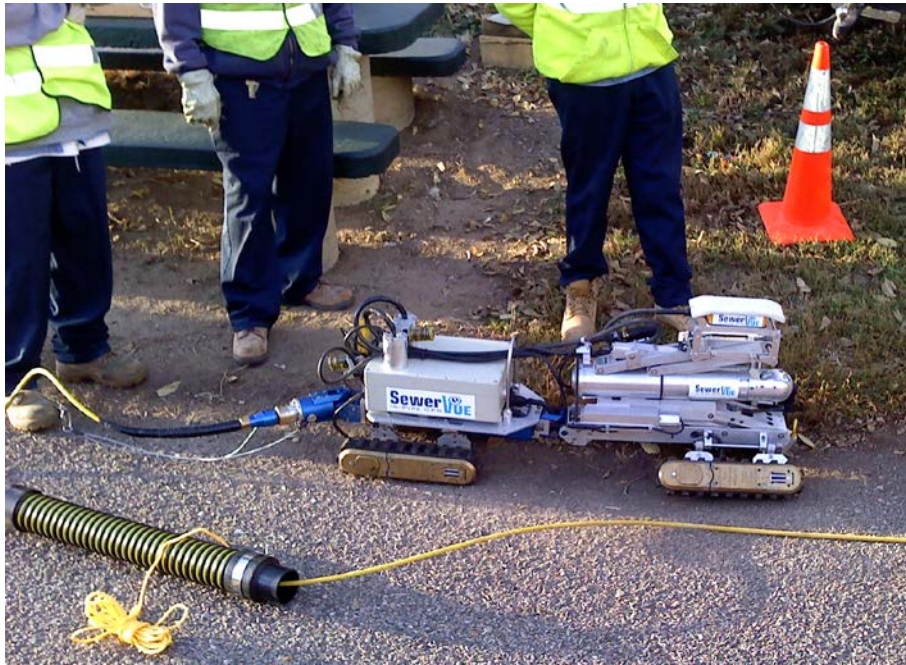
Figure 3. Metro Wastewater O & M personnel readying the SewerVUE Surveyor robot for deployment at Harvard Gulch Interceptor, Denver, CO.
