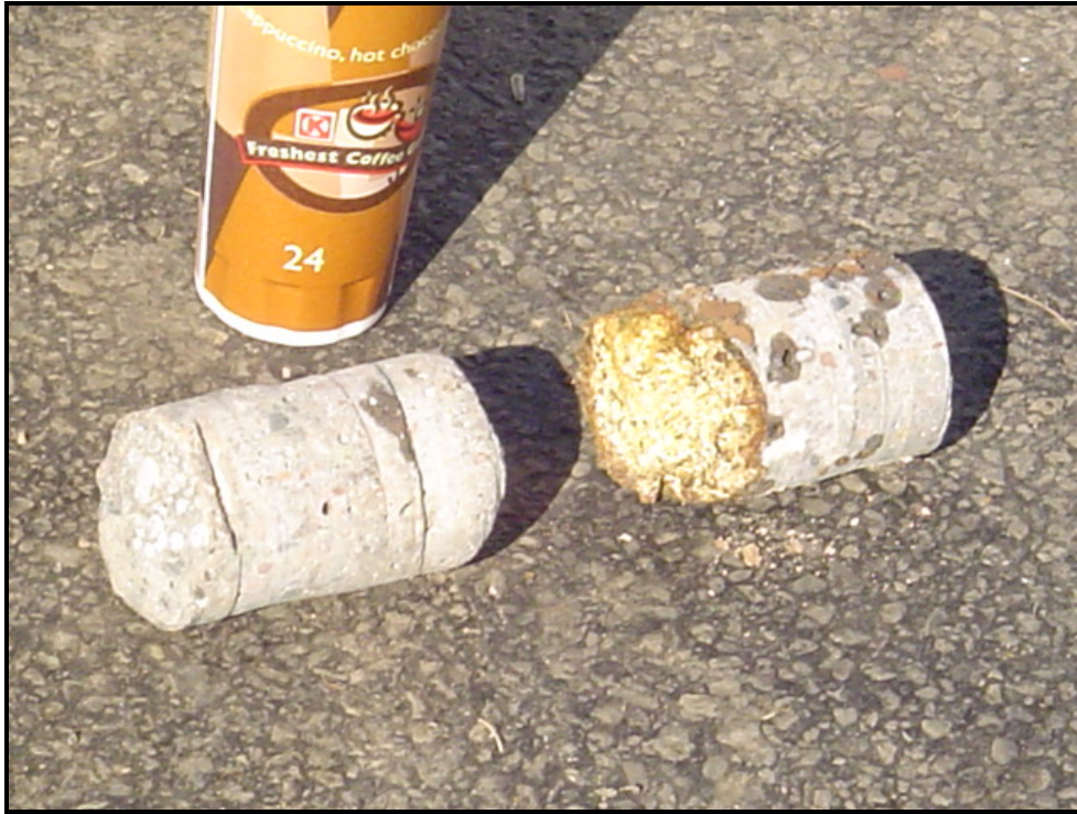
Figure 9. Core samples from 750 mm concrete pipe section
