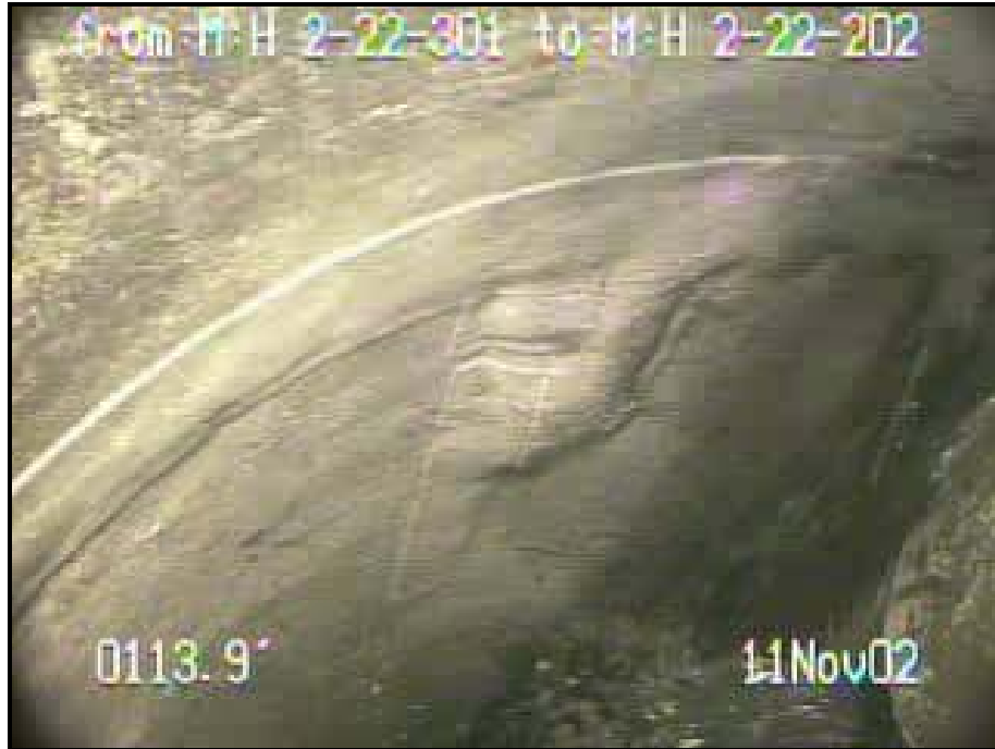
Figure 4. Blister in liner
