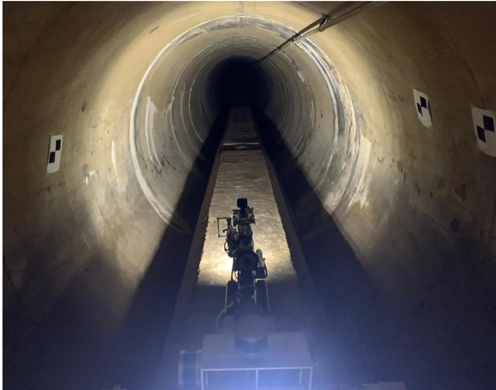
Figure 2. SewerVUE Surveyor at top of the box culvert inside the 3000 mm storm pipe
