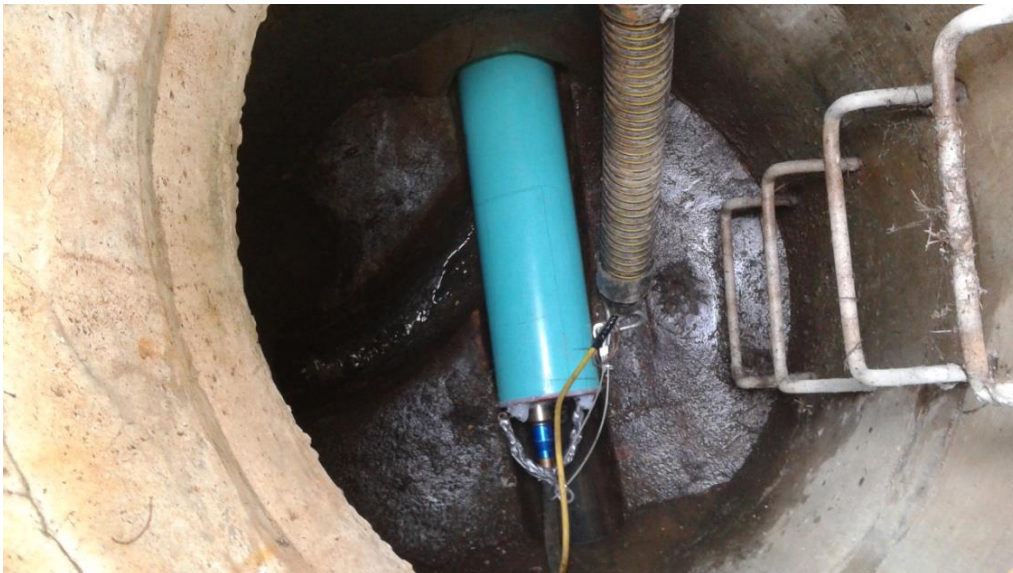
Figure 5. Deployment of the AC Pipe Scanner at the Harbourgreene drive sewer in Surrey, BC, Canada.
