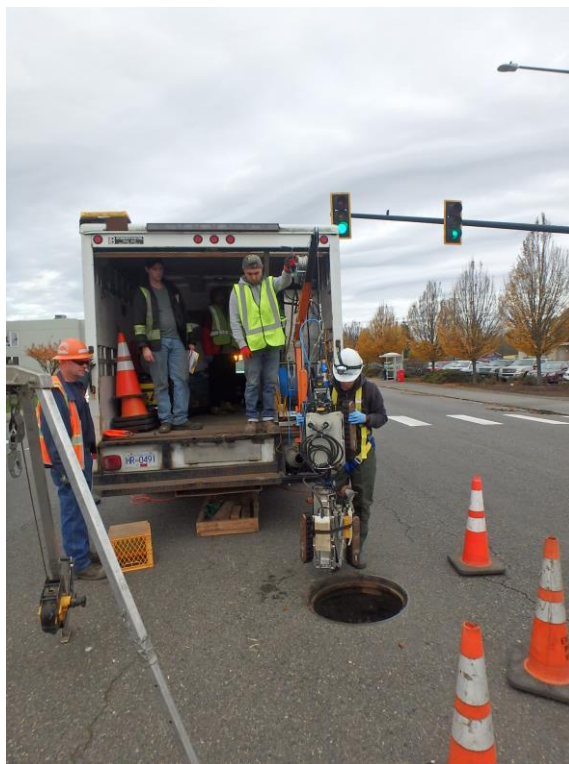
Figure 3. Deployment of the SewerVUE Surveyor robot at the Broadway Sewer main, Everett, WA.
