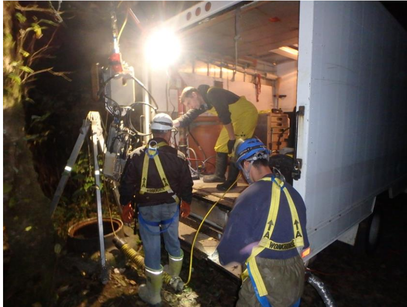
Figure 3. Technicians preparing for deployment of the SewerVUE Surveyor at the Bear Creek Trunk Sewer in Surrey, BC, Canada.
