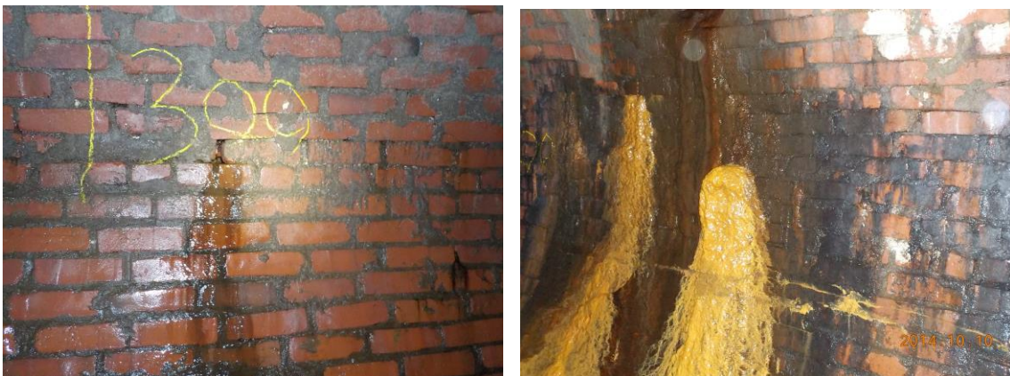
Figure 8. Visual observations such as infiltration or clay deposition were recorded during the inspection. Most of the pipe visually appeared to be in a good condition.
